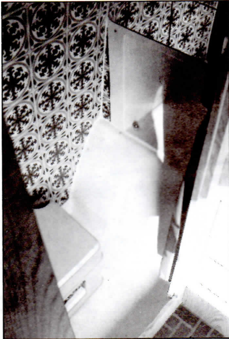
Details of toilet compartment. Note alcove for storing toilet when taking a shower.
